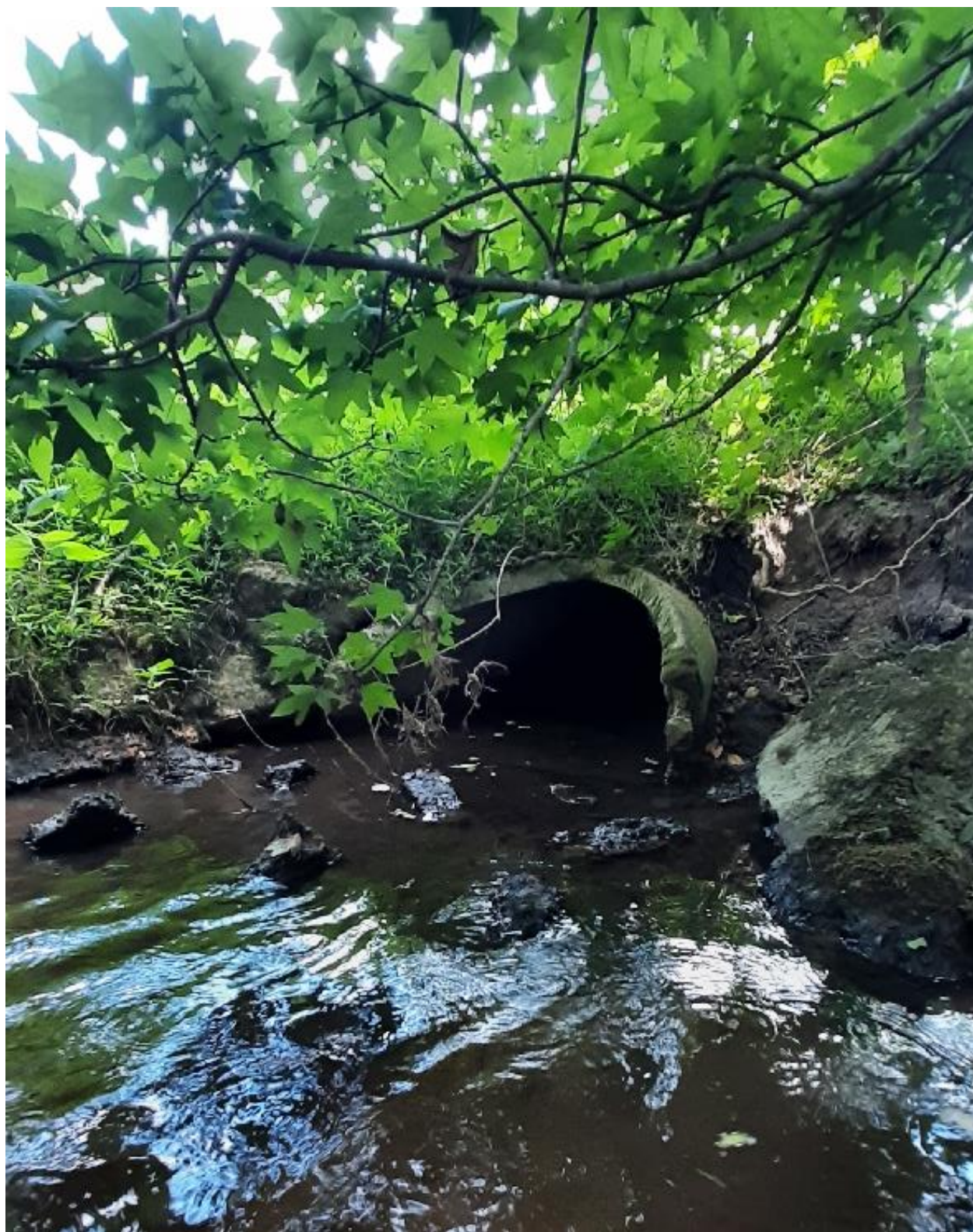
Outfall ID: MR23 (7/21/2022)
