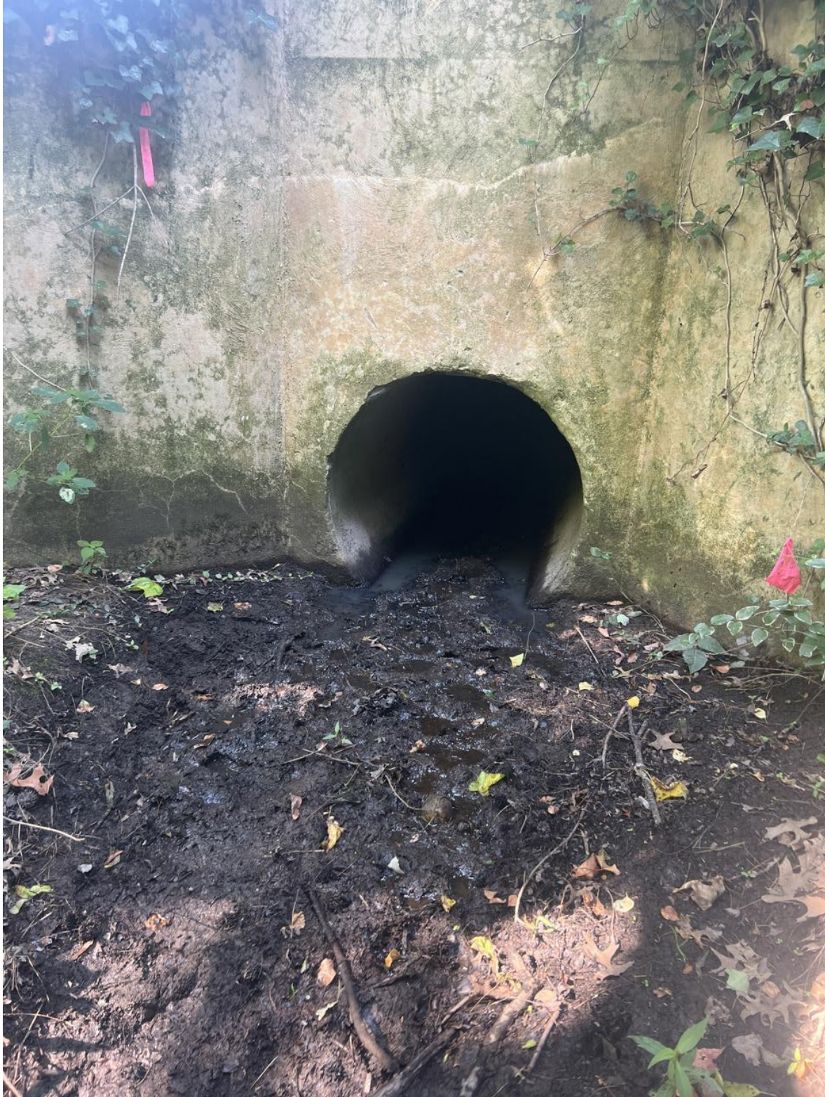
Outfall ID: MR06 (7/22/2022)
