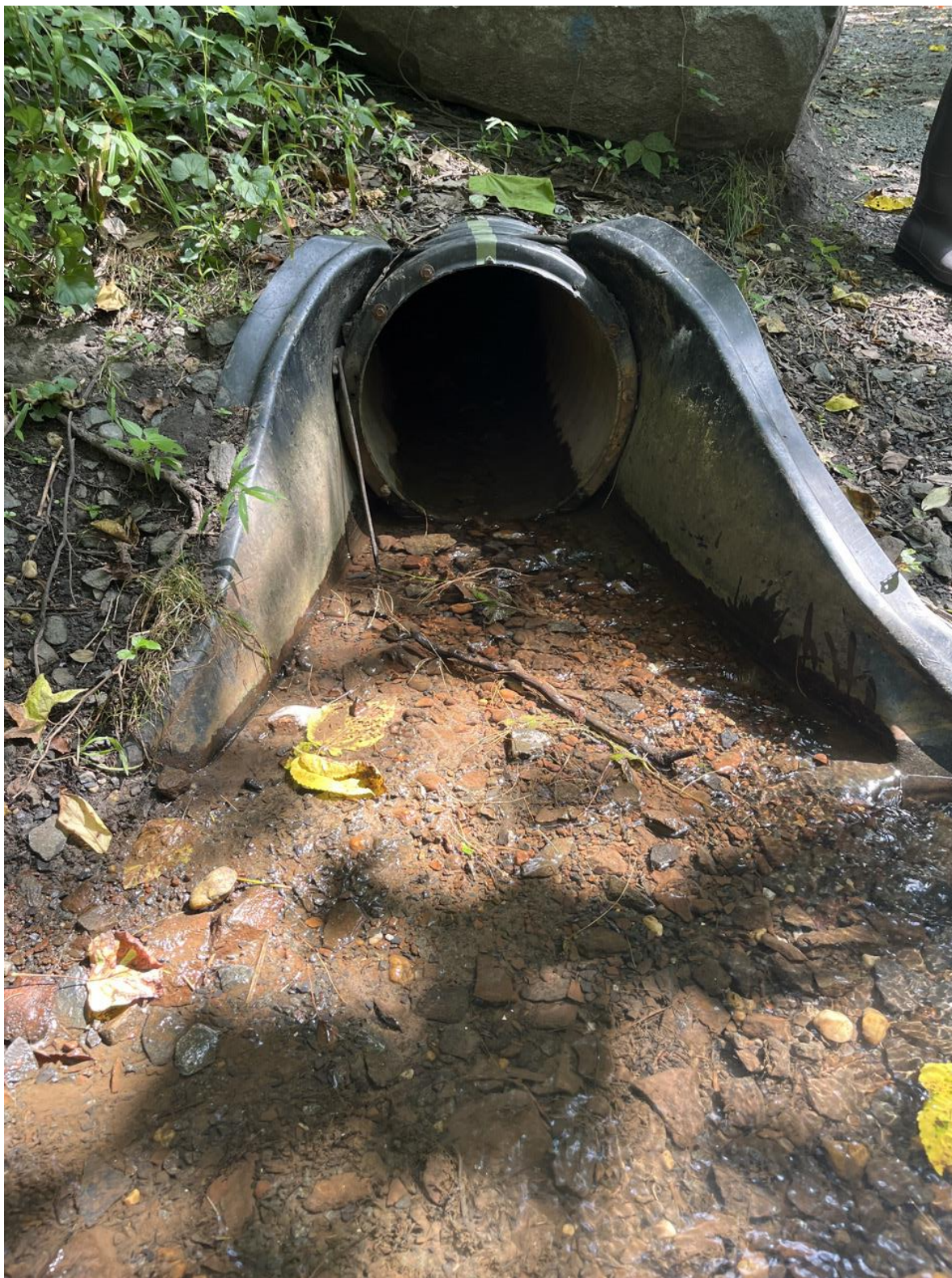
Outfall ID: MR19 (7/21/2022)
