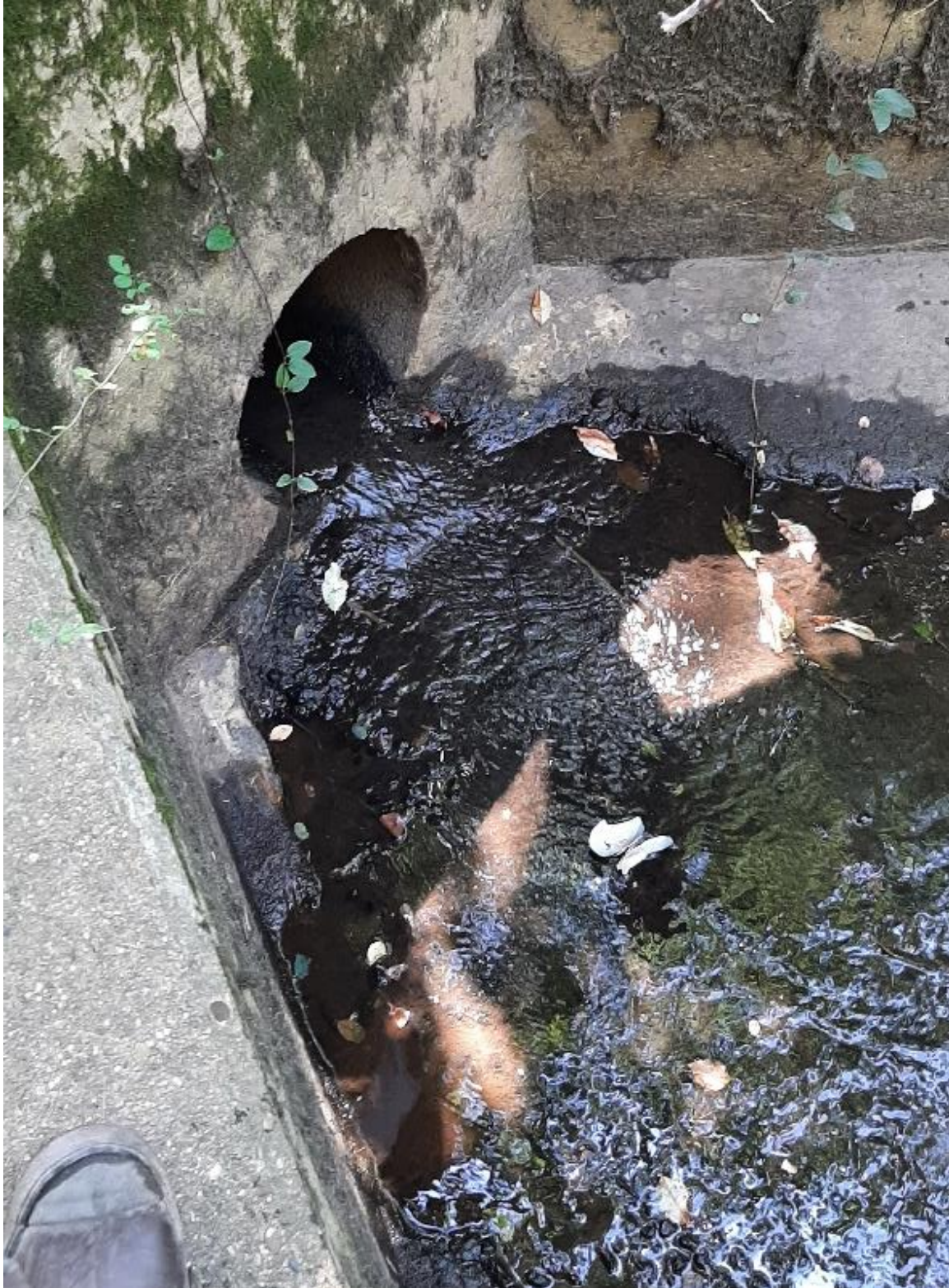
Outfall ID: MR13 (7/21/2022)
