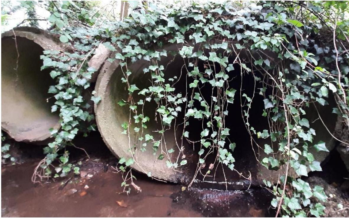
Outfall ID: MR25 (7/21/2022)
